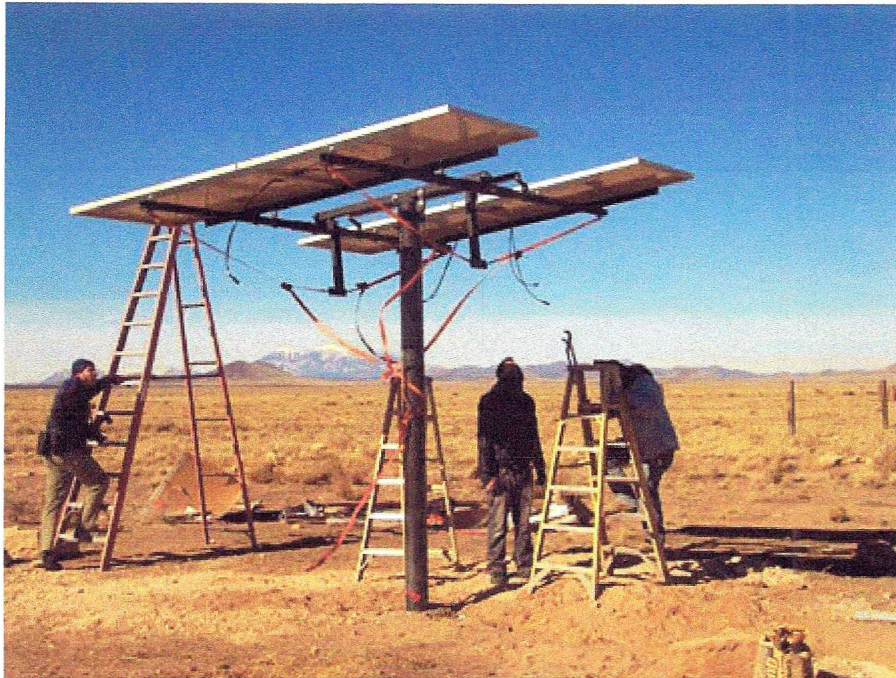
A solar tracking system provides electricity to the EMPUS
