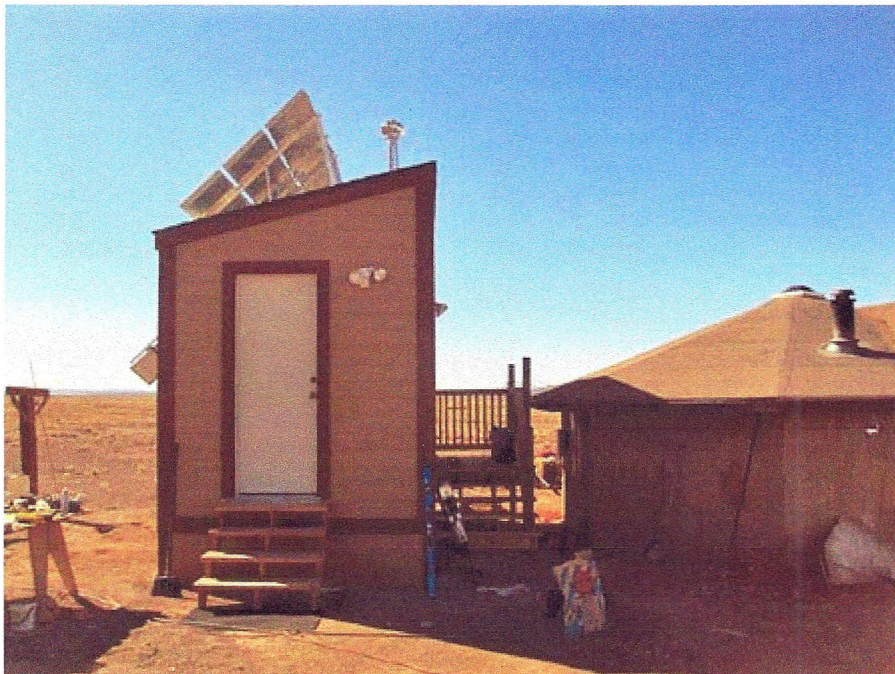
The stand-alone utility building, called the EMPUS, will provide heat, electricity and hot water to the tribal Hogan, with a hallway connecting the two
