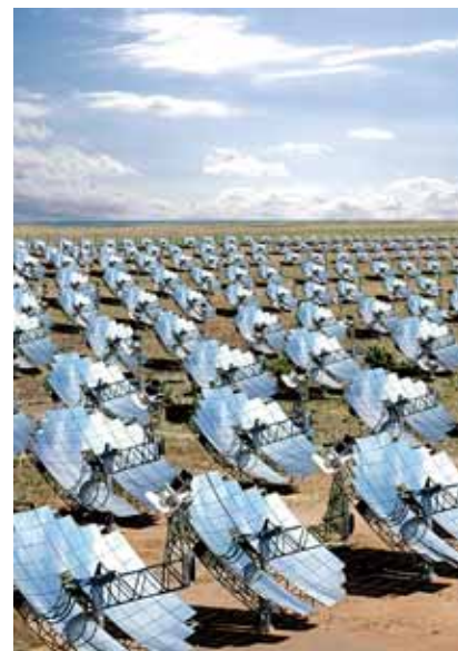
Stirling Energy Systems SunCatcher solar farm for the Imperial Valley - Southern California
