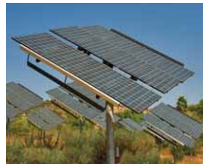
Example of a local PV tracking system used at Alpine Elementary School (independent of SDG&E)
